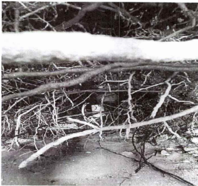
Broken irrigation valve/pipe in cavity under sod
