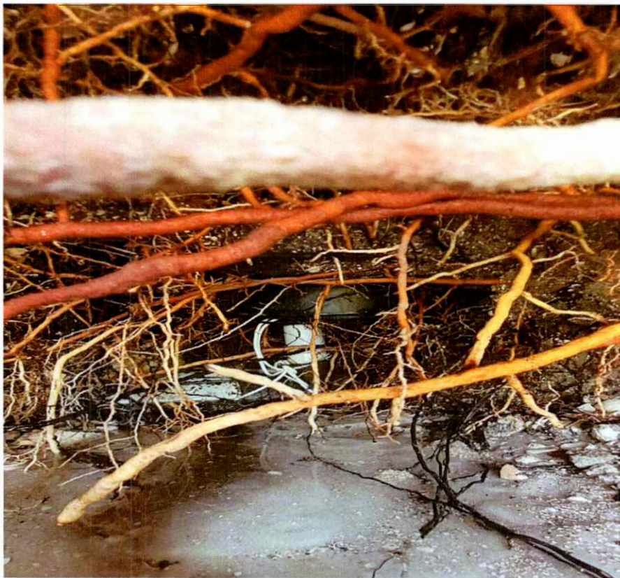
Broken irrigation valve/pipe in cavity under sod
