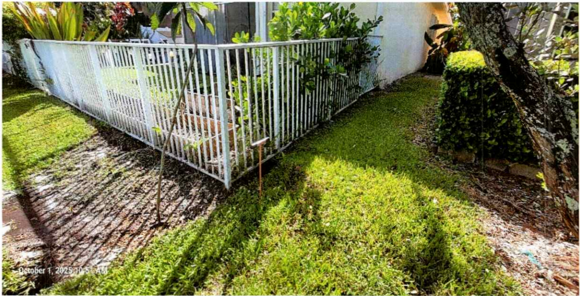
Orange Stake location of irrigation valve/leak
