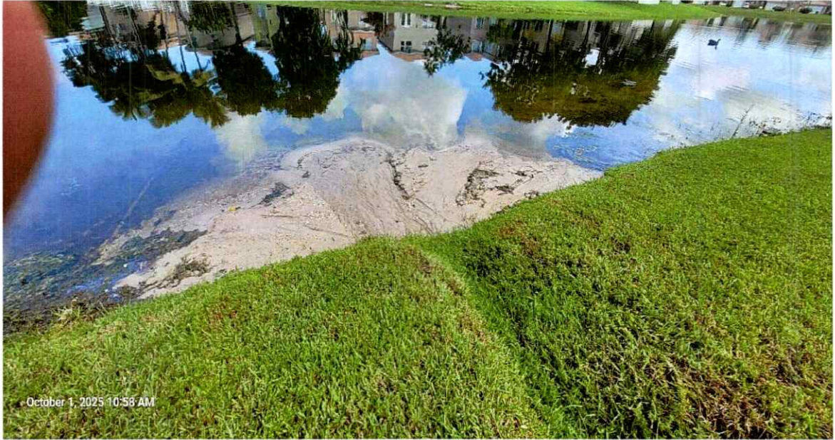
Sand washout into lake 9
