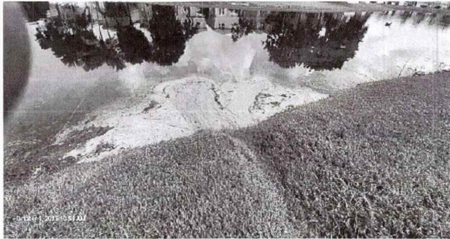
Sand washout into lake 9
